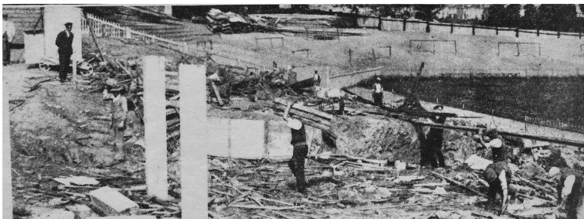
Demolition of the Home Park wooden grandstand complete. (Western Morning News, 17 th June 1930).
